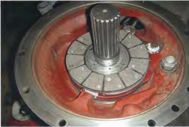
Brake plates and brake anchor plates were replaced into the axle shafts.
